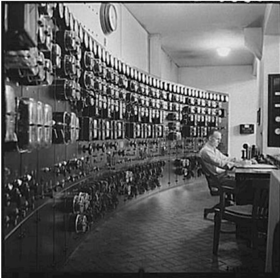
Figure 1: Control room, waterworks. Conduit Road, Washington, D.C.
